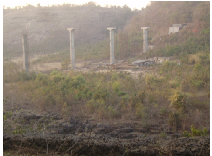
Photograph 4 BRIDGE WITH TALL PIERS Spanning arrangement: 8 spans of 47.5m Clear roadwidth+Road+Crash Barrier: 12.75m (2Lane) Dead Load:1200t Live Load: 90t
